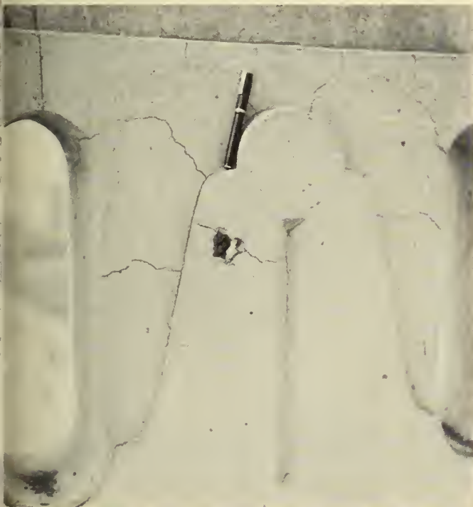
FIGURE 7. Popout around opaline shale fragment, Sixth Street Bridge, Los Angeles.
